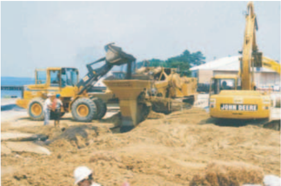
FIG. 7. (a) Continuous trenching machine used to install the 46 m long, 7.3 m deep and 0.6 m wide granular iron permeable reactive barrier; (b) simultaneous excavation and replacement of aquifer material with granular iron as the horizontal trencher advances [193].
